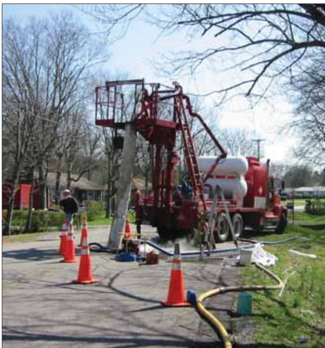
The project involved 94,000 lf of CIPP ranging from 8 to 24 in., the rehab of 415 manholes and renewal of 860 service laterals.
